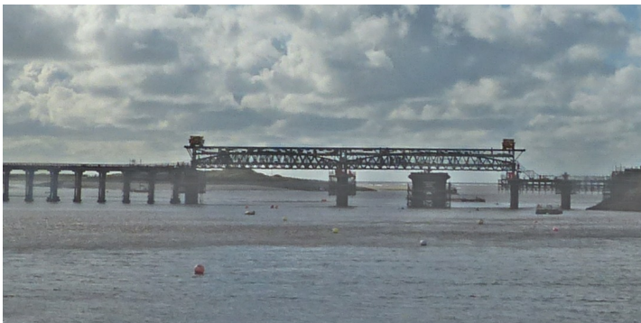
Barnouth Bridge in 2020 (above) and during the replacement of the two steel spans on 14th October 2023. Photographs Denis Bates
